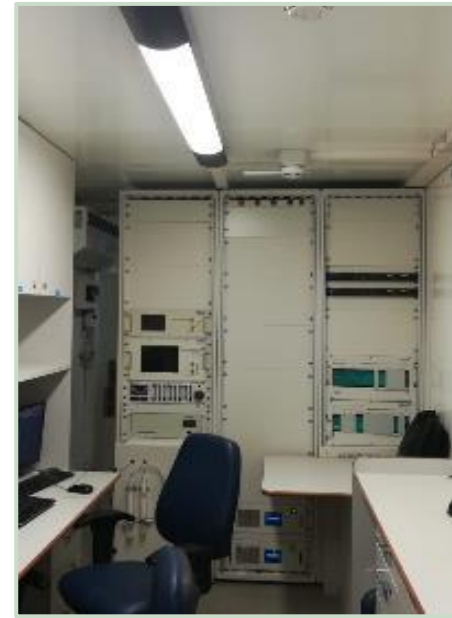
Mud Logging Unit
